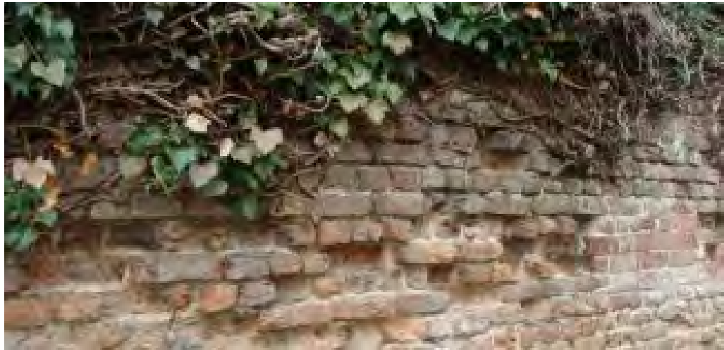
Picture 1.32 Boundary wall to Audley End Estate, an important feature and in urgent need of repair
