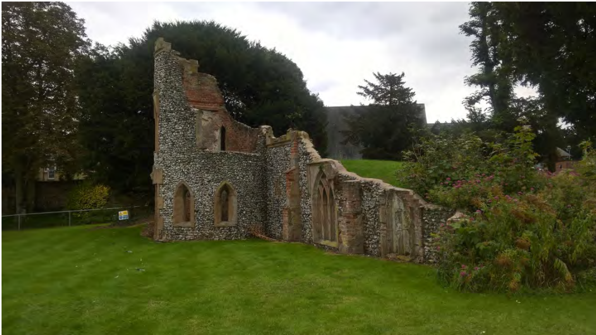
Picture 1.19 The Folly, Elm Grove - A Grade II listed structure which has benefitted from consolidation works and repairs.
